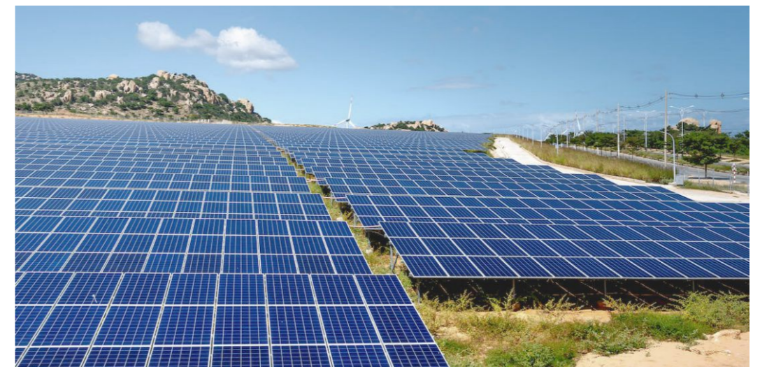
1.3MW Ground-mounted PV Plant
