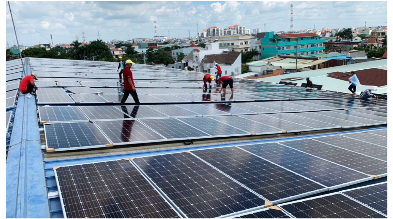
443 KW Rooftop Power Plant
