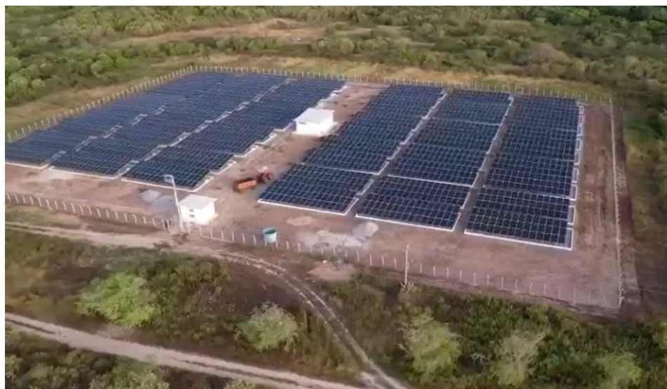
2.1MW Ground-mounted PV Plant
