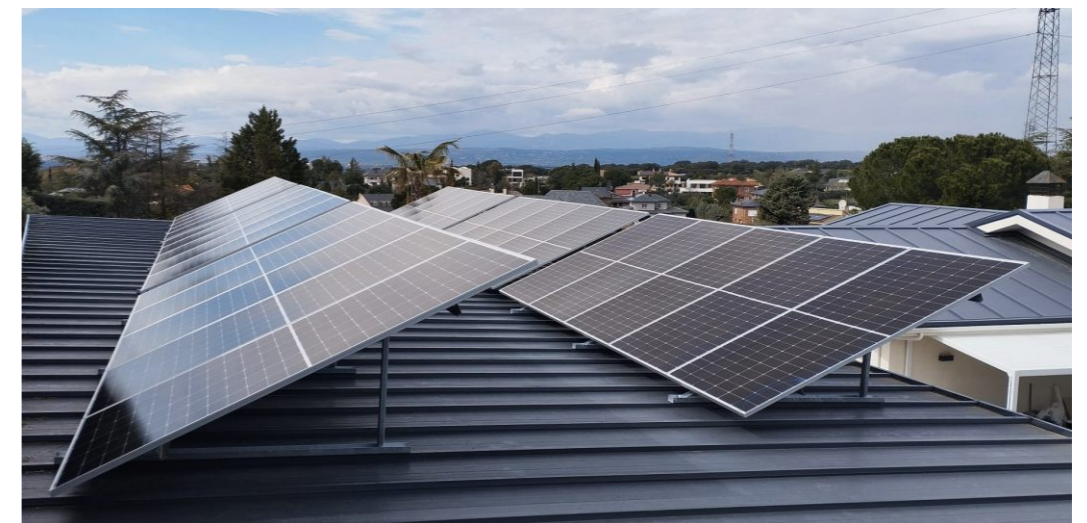
17.4KW Rooftop PV Plant
