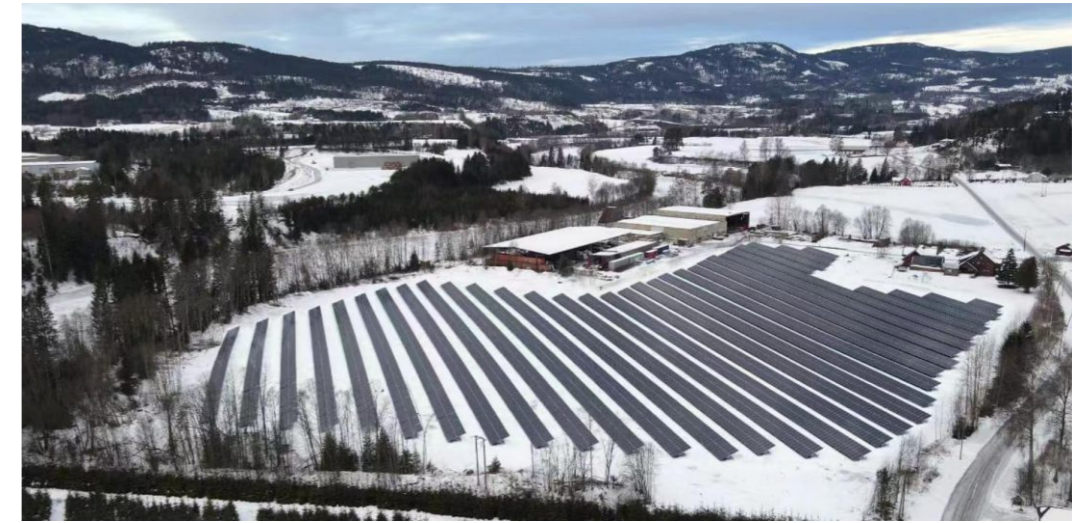
6MW Ground-mounted PV Plant
