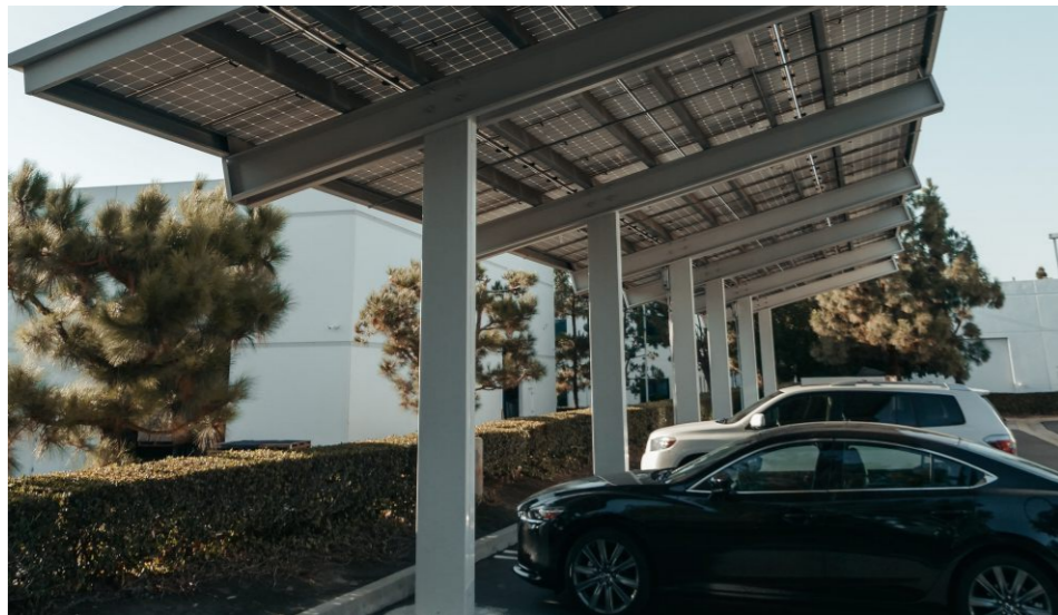
65KW Carport PV Plant
