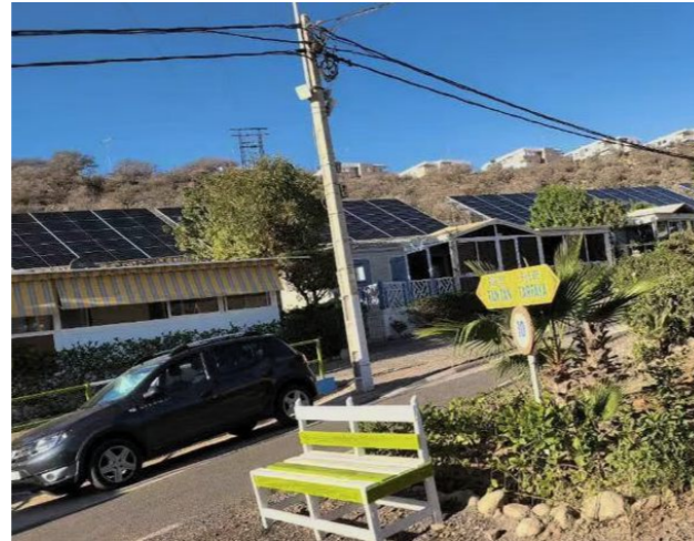
3MW Rooftop PV Plant
