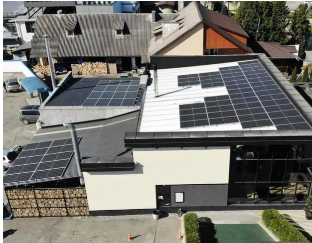
40.25KW Rooftop PV Plant
