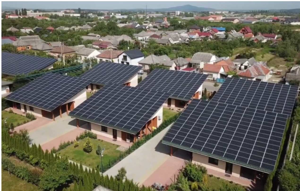
550KW Rooftop PV plant
