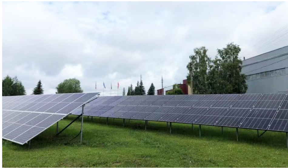
80KW Ground-mounted PV Plant
